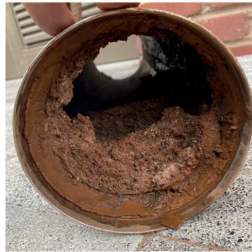
Figure 1: A 40µm filter basket from a reaction tank (as in Figure 3) that was removed shortly after installation into a new-build system
