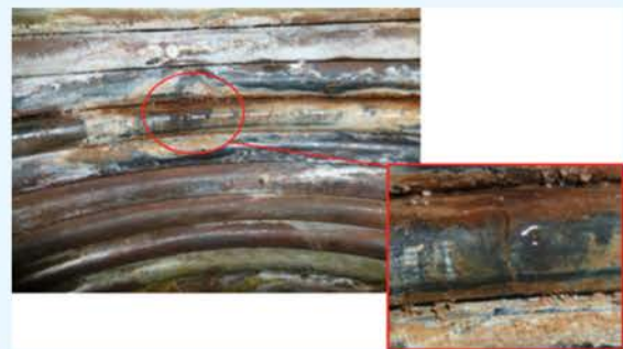
Limescale on surfaces lead to high temperature differences in the heat exchanger itself - thermal stress causes cracks with leaks.
